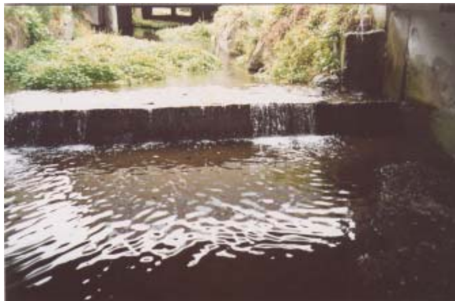
Figure 12: Korokoro Stream. A 0.6 m high weir that would restrict inanga to habitat below this point. Suitable spawning vegetation was downstream of this structure.
