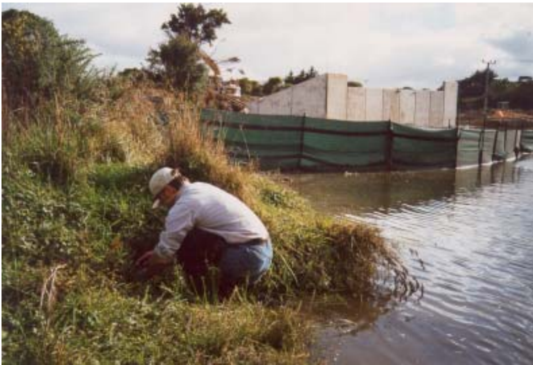
Figure 31: Suitable inanga spawning habitat just upstream of the new bridge over Pauatahanui Stream, on the true left bank. Note the measures to control topsoil runoff around the construction site.
