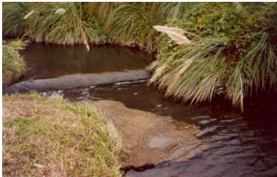
Figure 26: A low weir on Kenepuru Stream that did not appear to serve any perceived purpose. Such structures are best removed, if they are obsolete.
