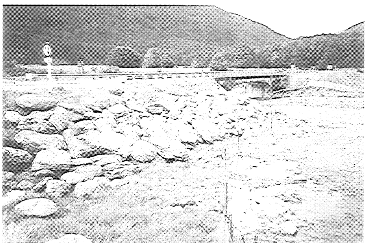
Camerons Creek Road Bridge after the January 1994 flood, with riprap protection. (From 'Bridge Scour', by Bruce W. Melville and Stephen E. Coleman, Water Resources Publications LLC)
