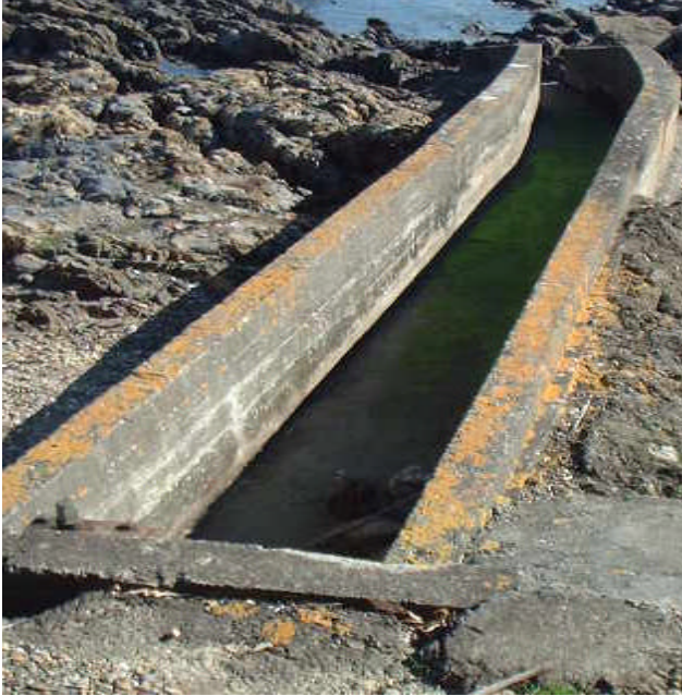
Figure 1 Emergency Sewer Overflow from Sorrento Bay, Eastbourne
