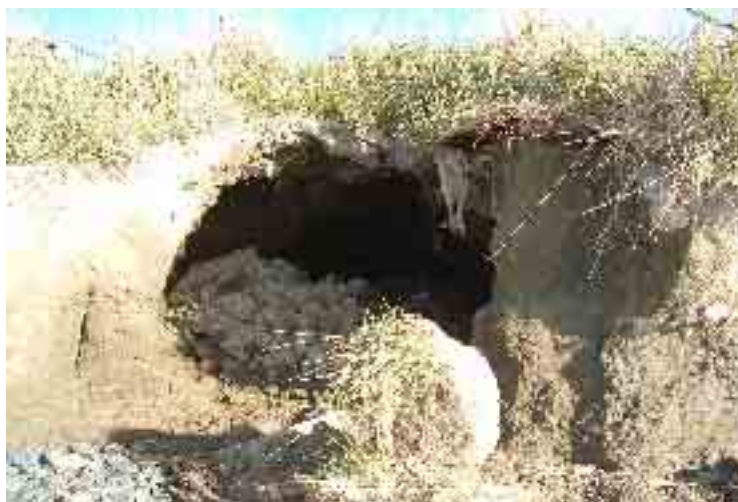
Figure 2: A large hole in the outer face of the Onoko Stopbank
