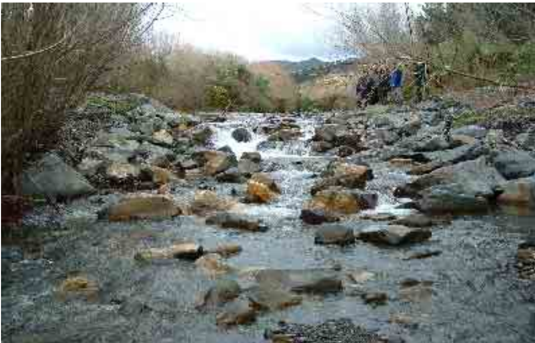
Figure 1: One of the Mongonui weirs, showing steps built to assist fish passage
