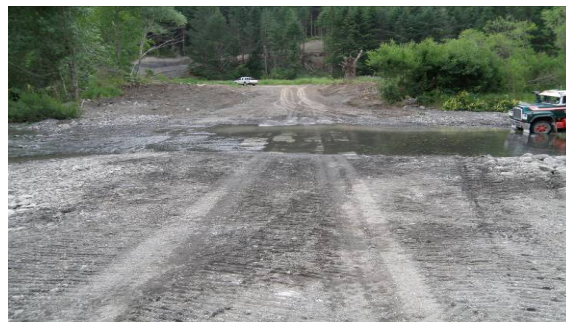
Photos of the Tauanui River ford made out of large concrete blocks
