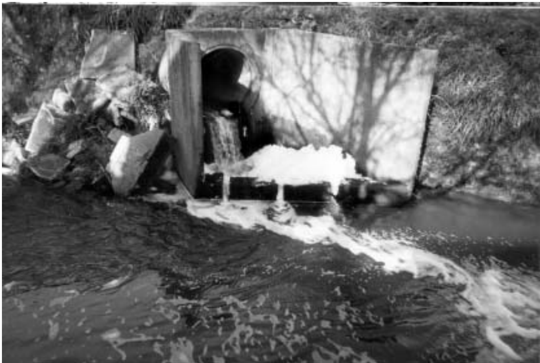
Figure 14: Foam discharging to a stream from a stormwater pipe, 30 July 1999.
