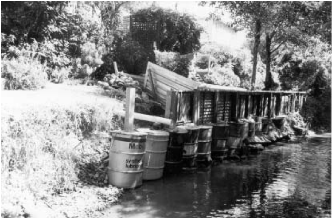
Figure 10: Unconsented bank protection works near Tawa, 9 March 2000.
