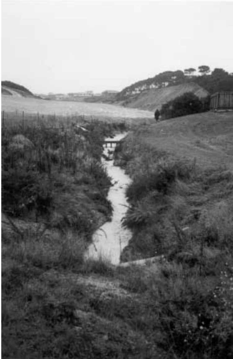
Figure 18: Subdivision works at Whitby Coastal Estates lead to silt discharge, 12 May 2000.
