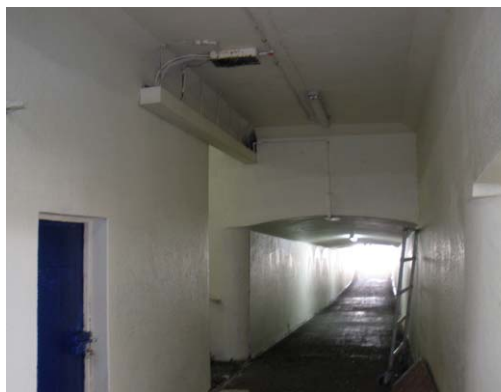
Before lighting upgrade
