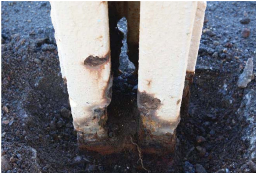
Figure 1: Corrosion of the footings
