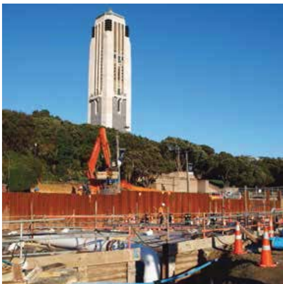
Above: Water supply pipework relaid as part of the Memorial Park development.
