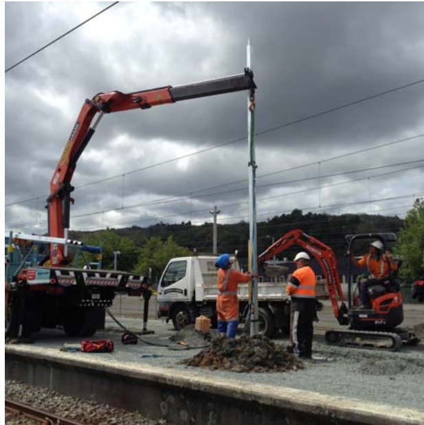
Fig. 1 New lighting poles being installed due to be switched on later this month
