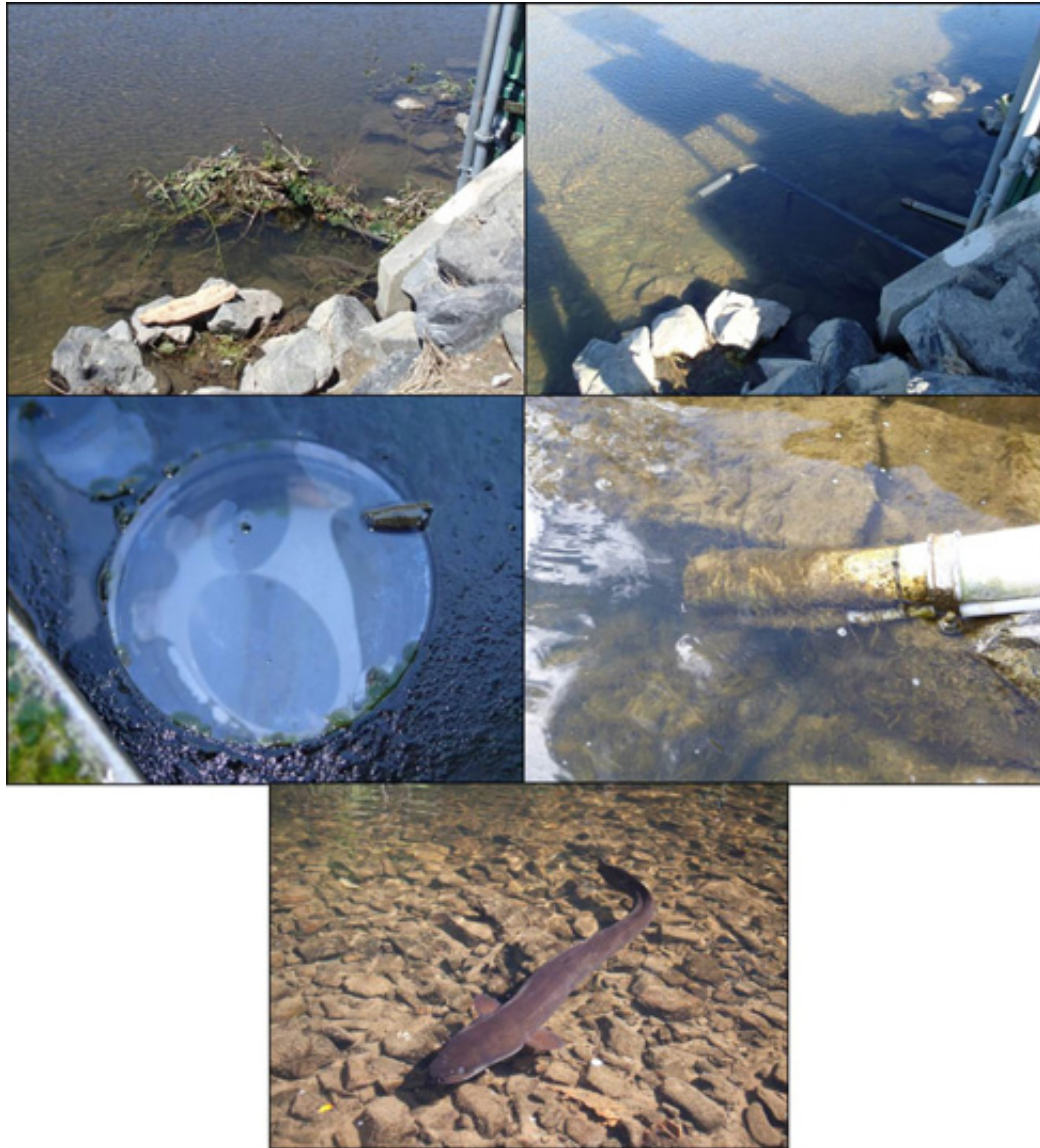
Figure 2.7: Examples of ‘fouling’. Debris snagged around the turbidity sensor housing at the Porirua site after a large flood in February 2013 (top left) and then the sensor again after the debris was removed (top right). A film of green algae which has built up on the edge of sensor lens at Porirua Stream (middle left) and filamentous algae growth on and around sensor housing at Horokiri Stream after several weeks of stable flow (middle right). Longfin eel which resides at the Pauatahanui Stream site (bottom)
