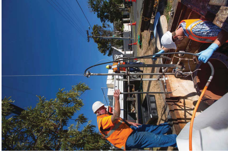
High pressure cleaning equipment is guided into a Knights Road well casing. The casing extends 39 metres down from the surface.
