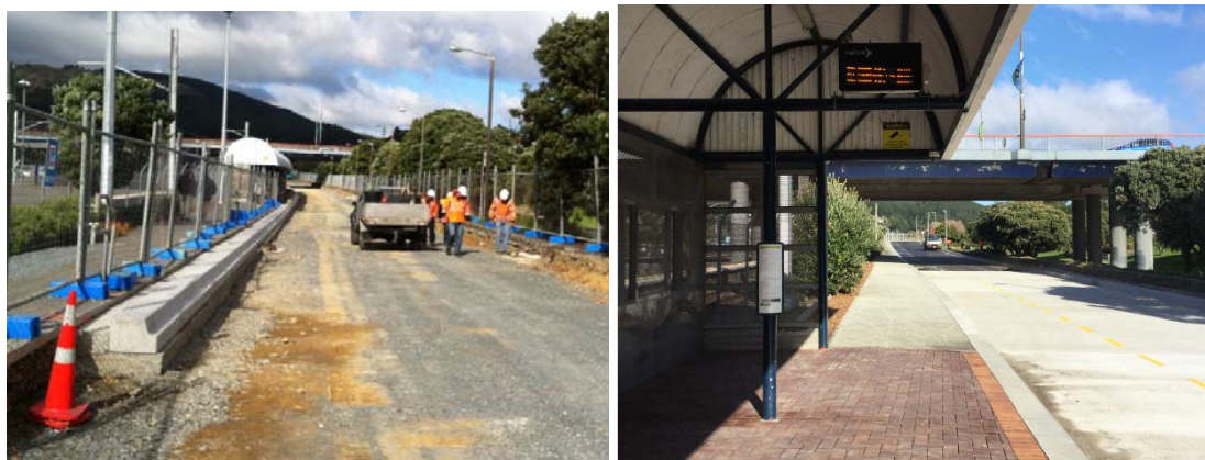
Porirua Station Road reconstruction, showing Kassel kerb installation (left), and work completed (right)
