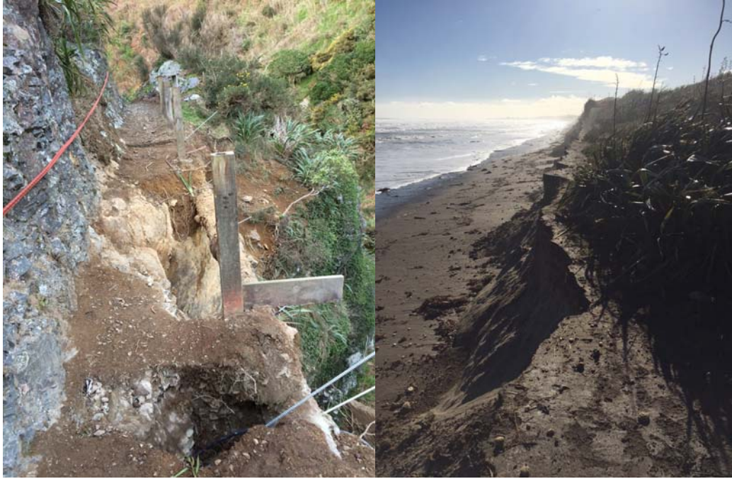
From left: Undermined Korokoro track; Coastal track washed away at QEP
