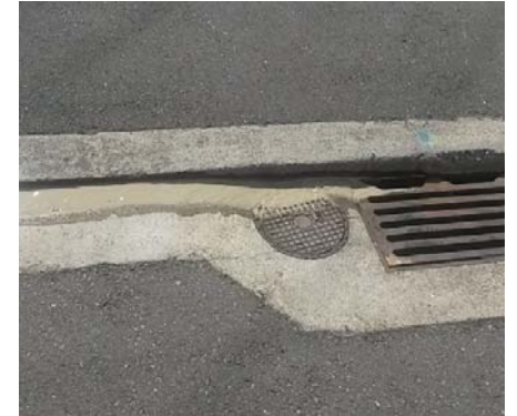
Cement washwater entering stormwater sump
