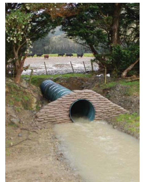
Unauthorised structure in a stream and discharge of contaminants to water
