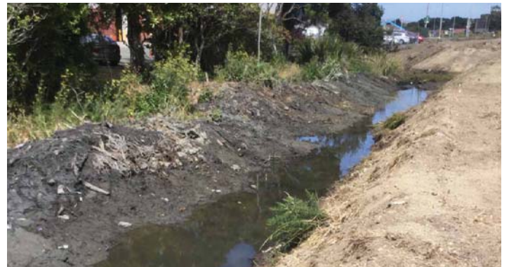
Figure 4: The unauthorised excavation of a stream which resulted in infringement
