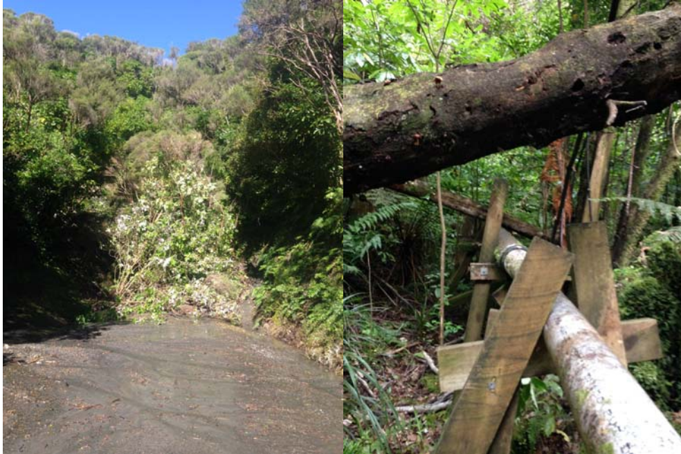
From left: Slip obscures Summit Tunnel; Tunnel Gully water supply pipeline
