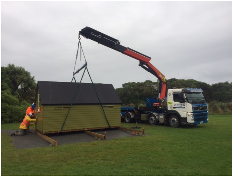
The newly restored hut is lifted onto its footings; sponsorship from Fletcher companies supported the MenzShed restoration work and transport to the park.
