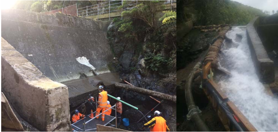
Contractors working underneath headwall to drill stabilising anchors ready for concrete pour; water diverted down spillway to enable repair, which will also provide for fish passage
