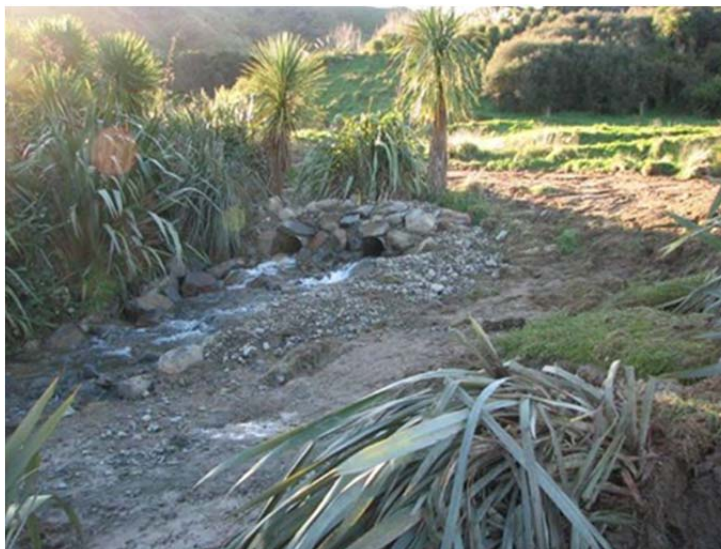
New rock ramp slows water flow and allows fish to move upstream
