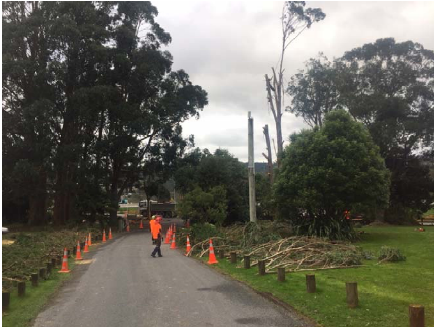
Tree removal underway; all gums to left and right of entrance gate to go
