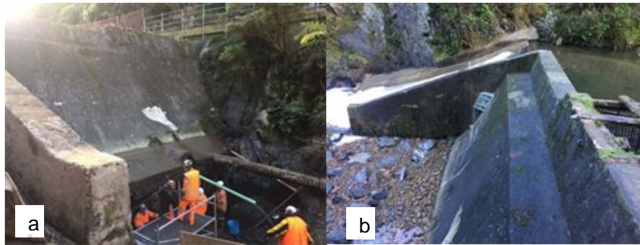
Woollen Mills Dam (Korokoro Stream) showing: a) the foundation repair-work in progress and b) the completed spillway repairs, shear bracket and scour protection work
