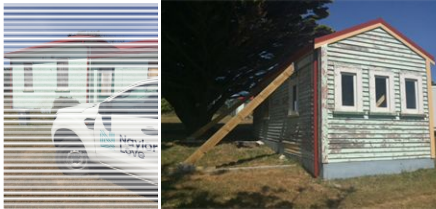
From left: generator building with new roof and spouting; historic garage with new roof, spouting and bracing.
