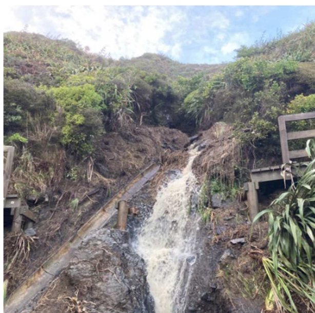
Figure 4. Slip above Culvert
