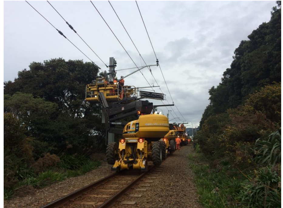
OHLE wiring run at Queens Birthday BOL
