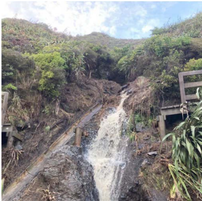
Figure 4. Slip above Culvert
