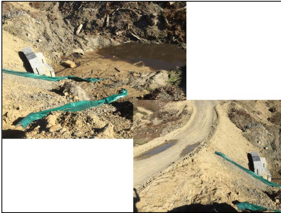
Letting the road drain straight into a stream where they have built a silt trap inside the stream
