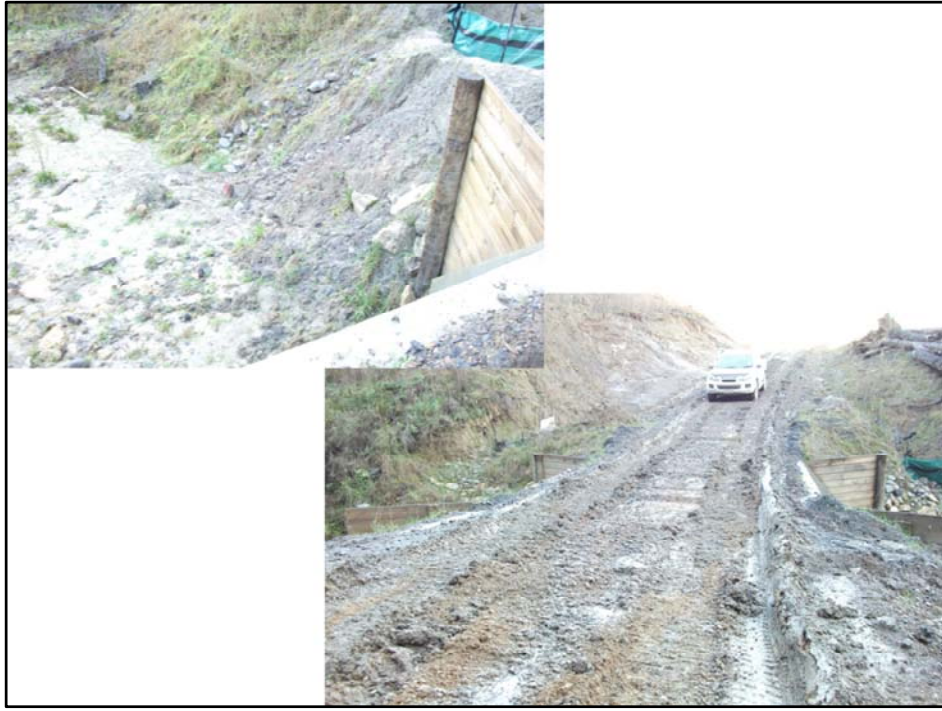
Poor sediment control on culvert let to sediment pouring into the river below
