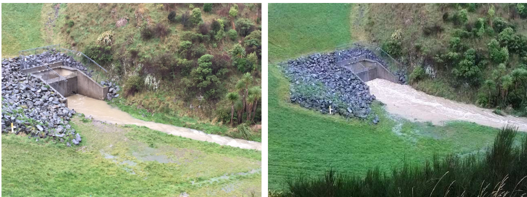
Figure 6: Stebbings Stream flood detention dam at Churton showing the energy dissipation structure at the outlet prior flooding (photos S. Miller) and after flooding in May 2015 (photos K. Neill).
