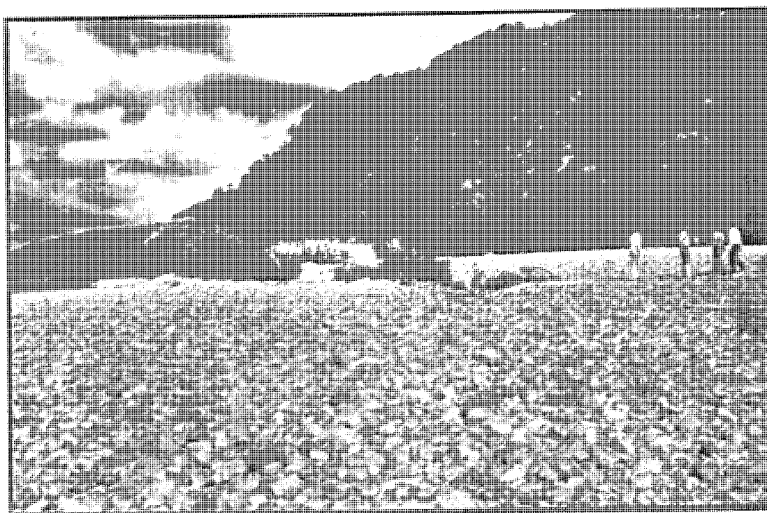
Plate 75: Failure of Silverstream Cut, c. 1984, showing the breach in the western bank protection works and the reactivation of the old western channel. Source: WRC photo.
