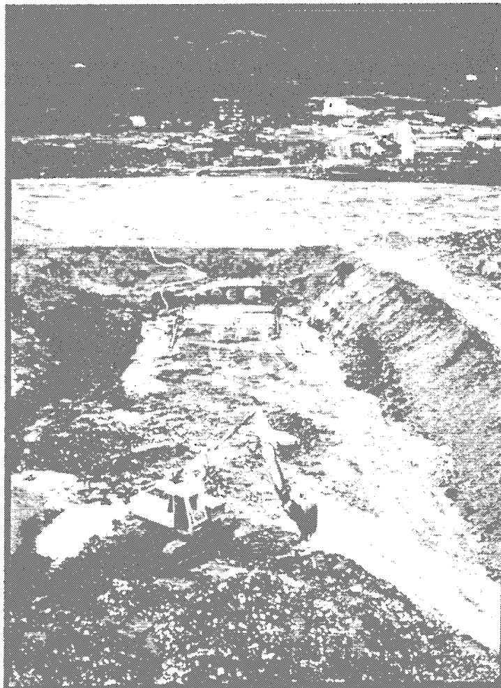
Plate 96: Construction of the sewer crossing 1976. Note the bed depth above the structure.
